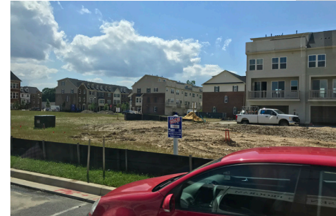
Construction is underway on 900 townhomes and 300 apartments at Greenbelt Station. Image Source: ULI Washington.
