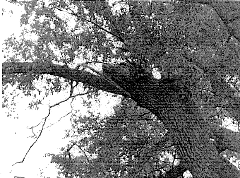
Stub from limb that appears to have recently split and fell onto building.
