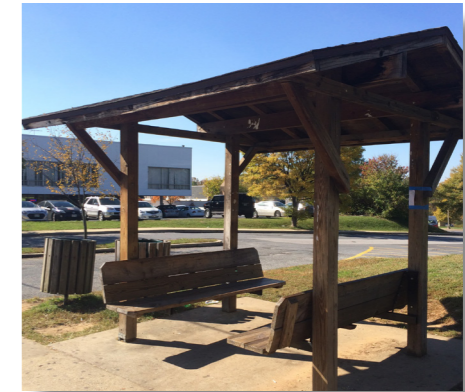
Existing bus shelter on Cherrywood Lane's west side near Beltway Plaza Mall.
