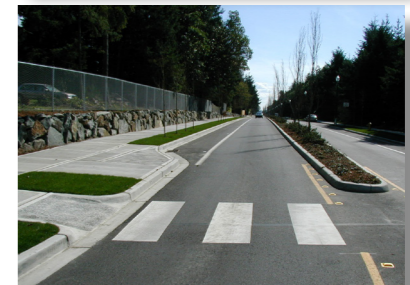
Options for improving crosswalk safety include refuge islands and striped or raised crosswalks.
